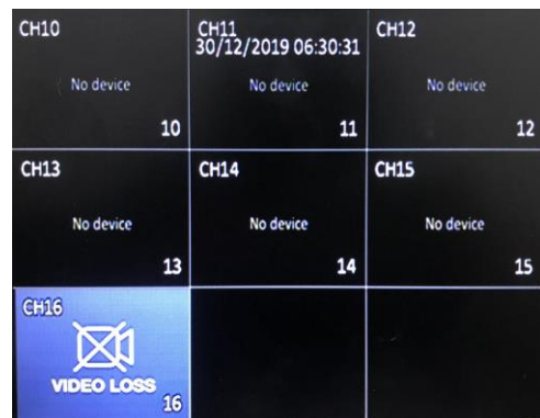
IP Camera Lost Data Connection Figure 6
